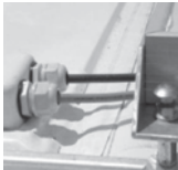
Option A: Using exiting cable entry point
